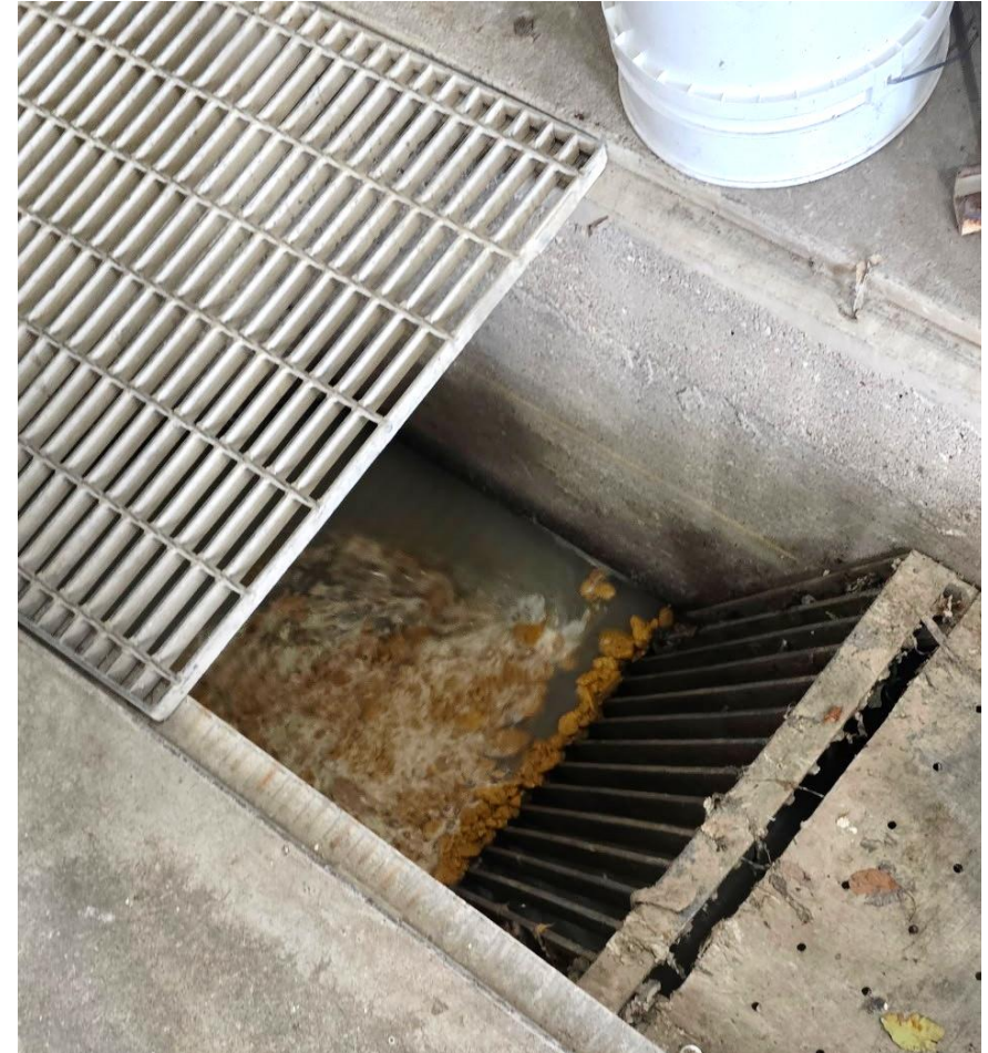
Grease flowing into the wastewater treatment plant on Oct 23, 2025.
